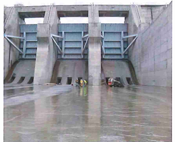
W.A.C. Bennett Dam spillway chute showing the three spillway gates, and the nine sluiceways containing slide gates, from the downstream side.
